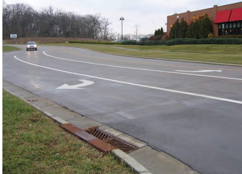
The City of Springboro drafted a capital improvement program aimed at upgrading all the concrete pavements at once.
