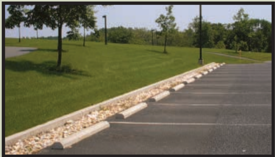
Figure 6 – In the event that the surface is repaved, an unpaved stone edge will still allow stormwater to reach the stone bed.
