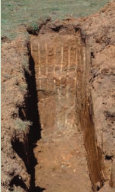
Figure 7 – Excavating a “deep hole” with a backhoe allows field investigation of the soils prior to construction.
