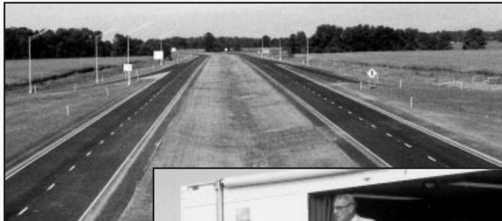
Relocated US Route 35 in Greene County looking west from SR 72. Prime contractor was Smith and Johnson with FPO member Valley Asphalt as the subcontractor placing the full depth asphalt pavement.
