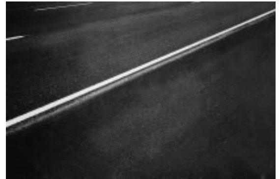
The SMA has successfully delivered the desired, distinct difference in texture and appearance between the pavement and shoulder surfaces.
