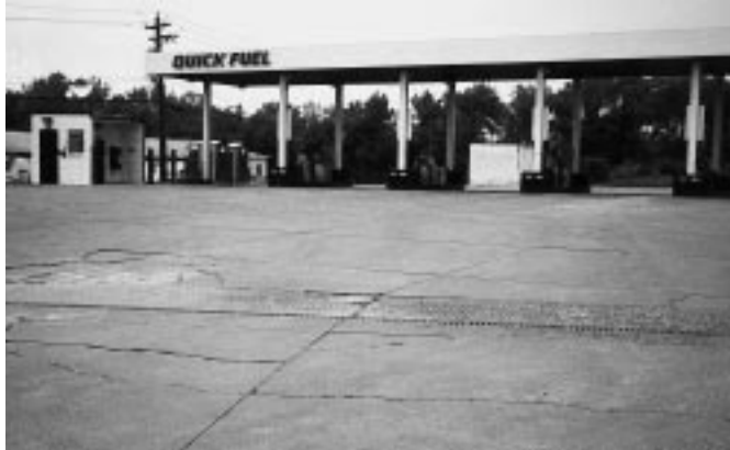
The original concrete pavement at the Sharonville Quick Fuel station required rehabilitation.
