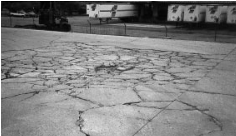
The pavement was heavily fatigued from the heavy truck traffic.
