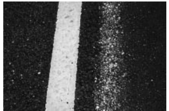
Coarse textured SMA on the left pavement surface, dense graded type 1 on the right shoulder surface.
