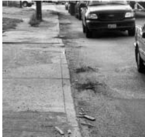
The existing asphalt surface on Broadway Street was severely deformed from traffic and distressed from age.
