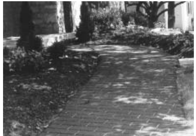
Asphalt also replaced existing concrete walk from driveway to front entrance and was finished in simulated brick to match drive.
