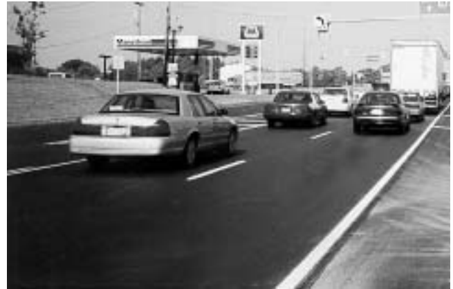
US 224 near Canfield receives treatment of 3/4-inch thick Type A mix (sold as SS 805). The project was constructed this August by McCourt Construction Company. Traffic on this pavement ranges from 20,000 to 36,000 vehicles per day.
