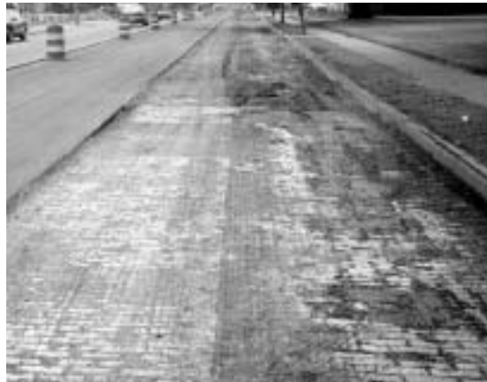
Severely distressed asphalt is milled to the bricks in the curb lane while the center lane is milled for a single course inlay.
