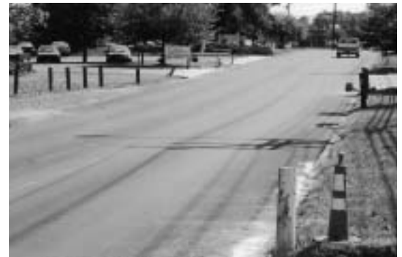
Creek Road traffic is maintained on the intermediate course while drive approach aprons are restored.
