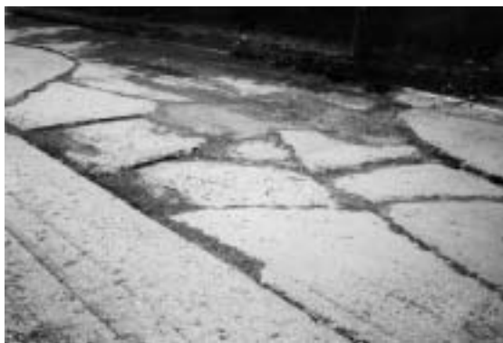
With the asphalt overlay milled off, the extent of the deterioration of the concrete base pavement was readily apparent.
