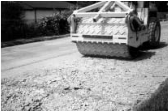
Rolling with a vibratory, z-bar roller further reduced the particle size and prepared the base for paving.
