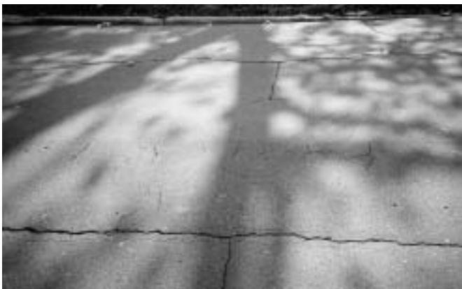
Type A surface mix on Shelburne Ave. continues to remain intact, resisting disintegration from reflective cracking.
