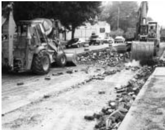
Removal of the bricks down to the 9-inch concrete base proceeded rapidly.
