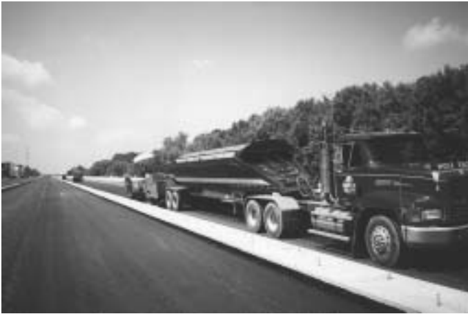
S.E. Johnson paving crew places big rock base course mix (302) for the Third Lane's paved shoulder.
