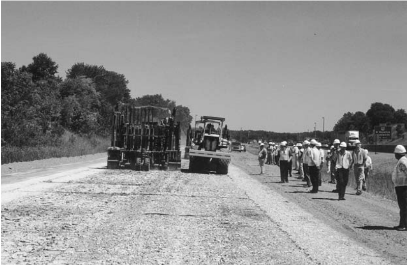
Concrete pavement on Medina 271 gets the rubblize and roll treatment while demonstration attendees look on.
