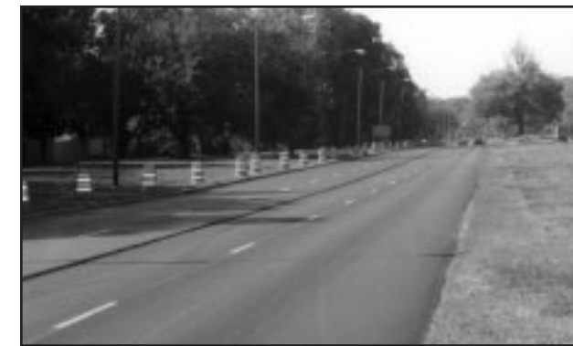
The Anthony Wayne Trail remains open to daytime traffic while waiting for the nighttime completion of the final surface course.
