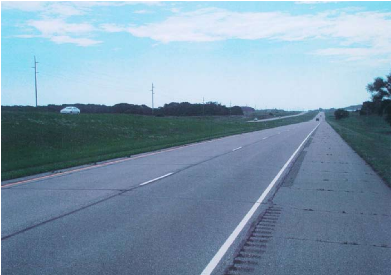
The Minnesota Department of Transportation won a 2009 Perpetual Pavement Award for the eastbound lanes of US TH 10, east of Detroit Lakes to east of Perham.
